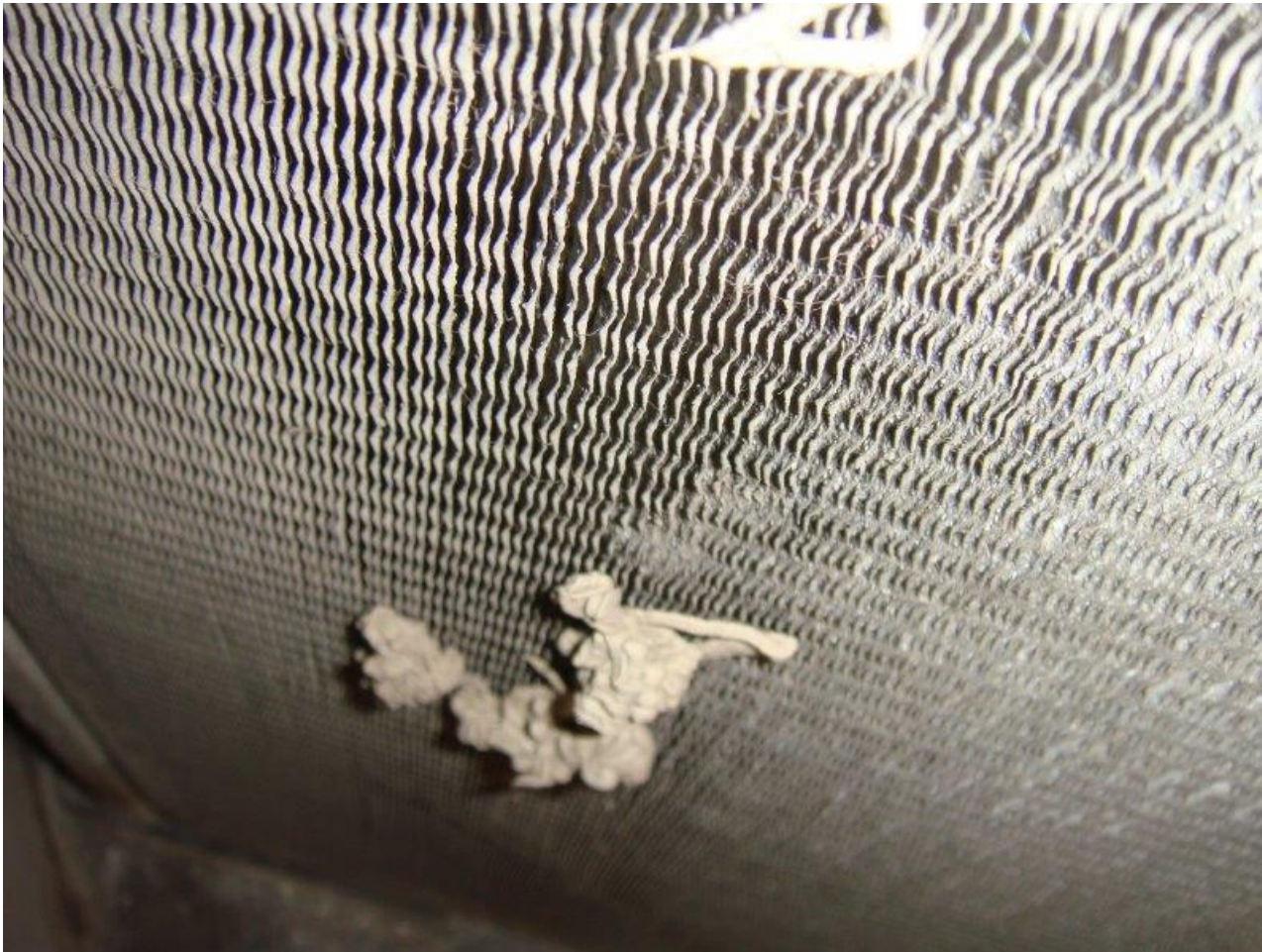
*Dirty condenser coil after CQM services
